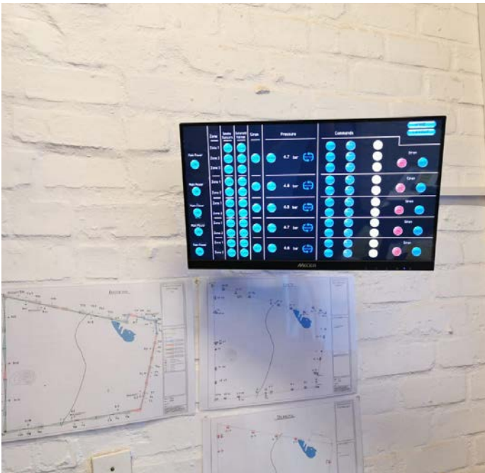
Commercial Wireless Control unit monitoring and managing multiple drencher units.
