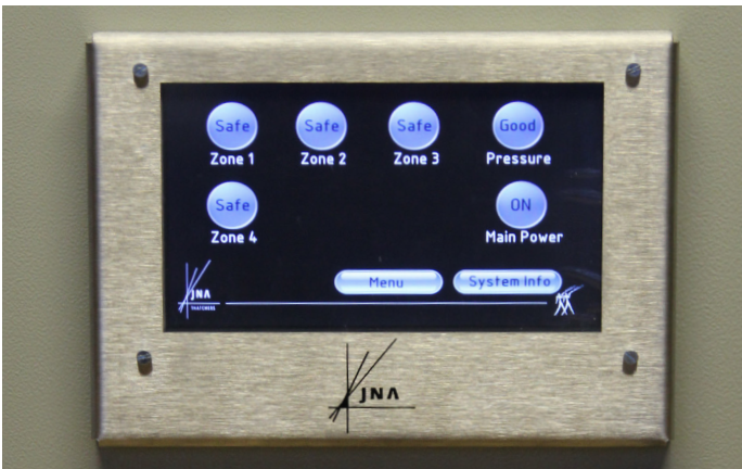
Cellular enabled drencher unit touch screen, showing zone status.
